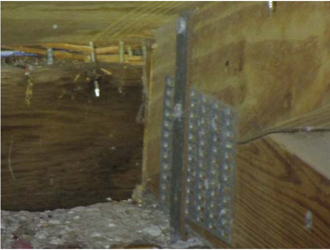
Toe nails - clips with only two nails
