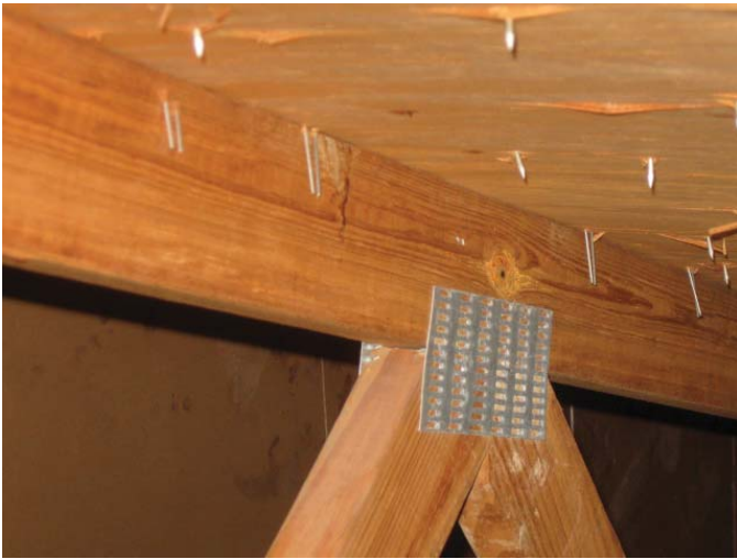
Staples no evidence of new renailling
