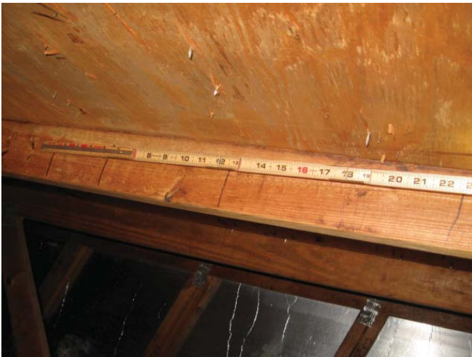
detection of metal spacing no evidence of new renailling
