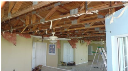
(Damage in Downstairs Unit)
